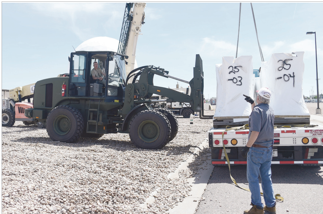
A construction crew unloads the new terminal a part of the Modernization of Earth Terminals project June 6 on Buckley Air Force Base. The MET project is replacing terminals installed from the 1980s with new ones in order to enhance the warfighters capabilities.
