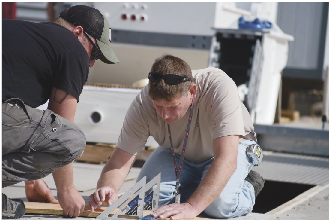
Construction workers measure out where to place the new terminal June 6 on Buckley Air Force Base. The new terminal will replace one that was installed in the 1980s. The new terminal will bring increased capabilities and communications options. U.S. Air Force photos by Airman 1st Class Luke W. Nowakowski
