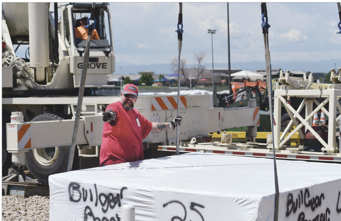
A construction worker guides a piece of the new terminal into place June 6 on Buckley Air Force Base. The installation of a new terminal is part of the Modernization of Earth Terminals project. The project aims to replace decades old terminals with new ones that enhance communications and capabilities.
